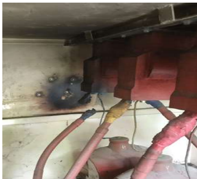
Servicing of 33 KVA Sub-station of new campus
